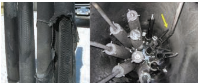
FIGURE 7. The ruptured coalescing elements and damaged riser support arm shown here were caused by excessive pressure drop across the vessel. Unfortunately, the pressure transmitter that should have provided an early warning of trouble malfunctioned due to below-freezing temperatures
