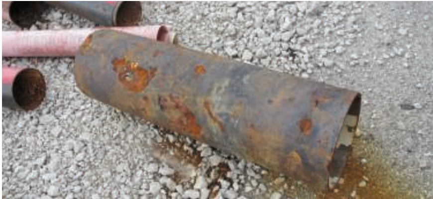
FIGURE 5. This sprinkler system pipe sat too long without flushing or oxygen scavenger maintenance. Premature failure was caused by grooving corrosion of the longitudinal pipe welds
